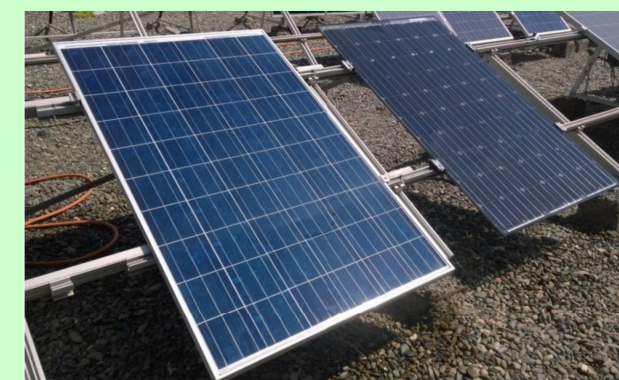
PV module installation at 25 degrees: Monofacial (left) and bifacial (right)
