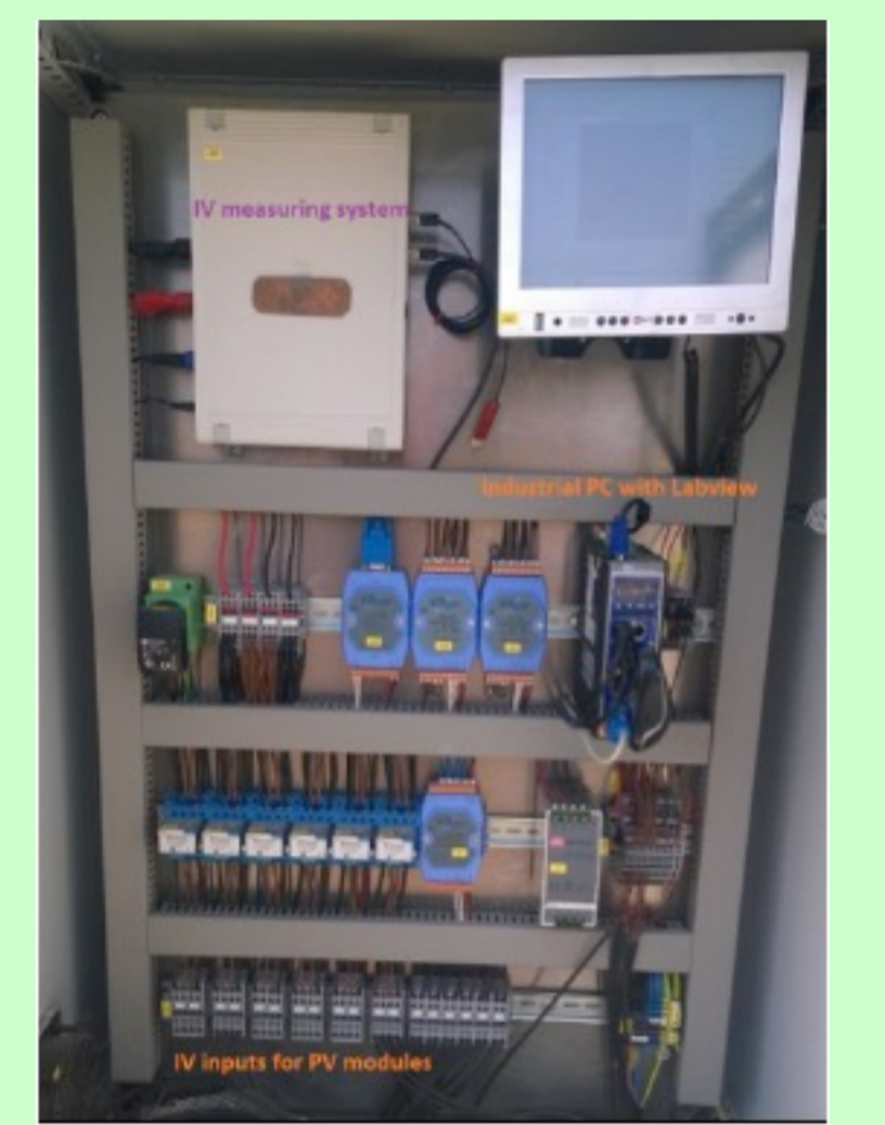
PV curve measuring system
